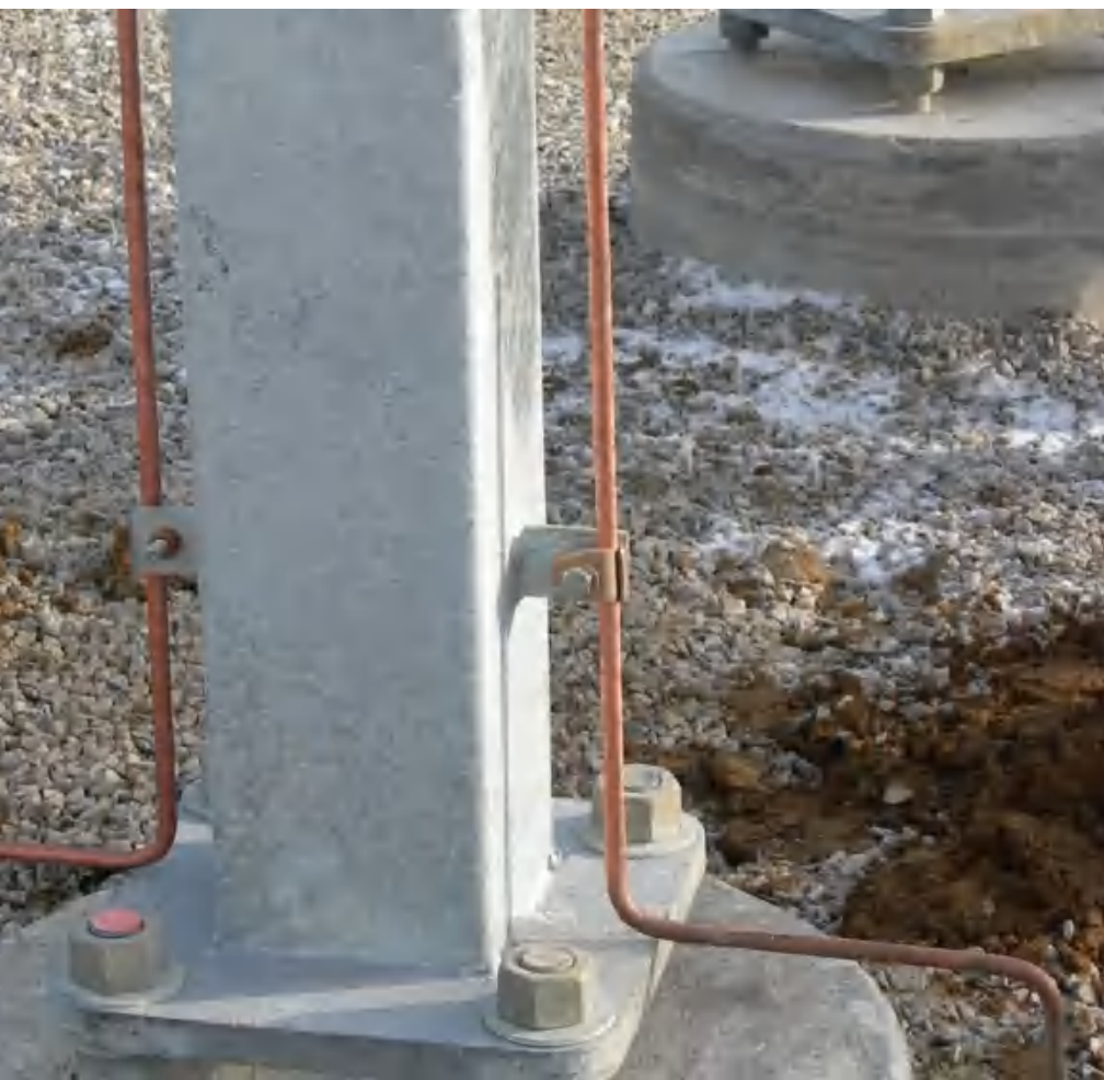
Substation earthing riser
