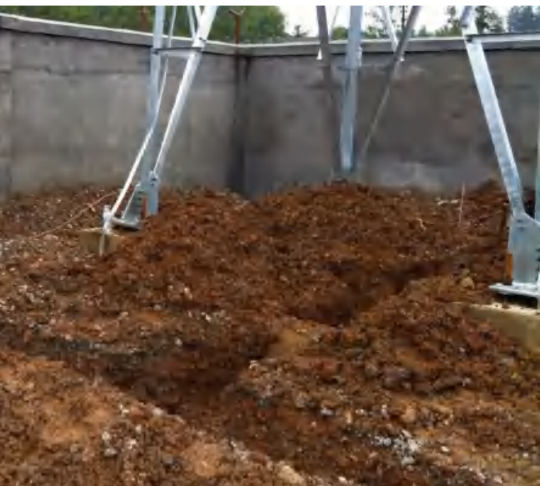
Telecom tower grounding
